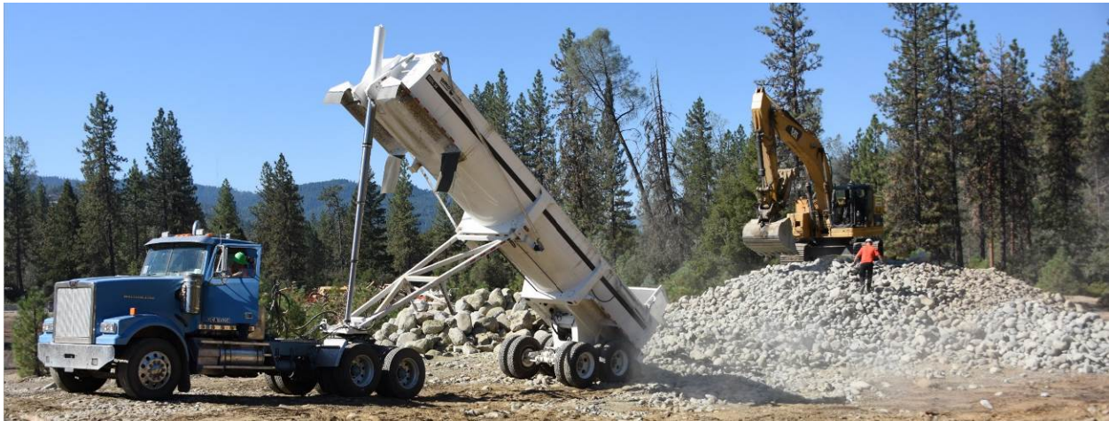
Figure 12. YTWRD crews processing gravel as part of the Trinity River Restoration Program.
