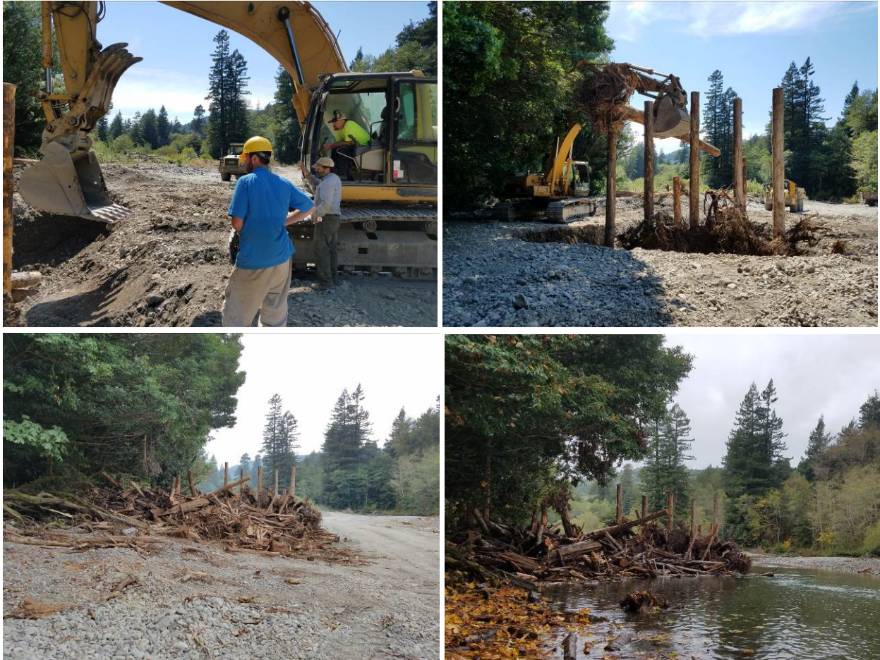
Figure 7. Photographs of wood loading activities in Terwer Creek (Top Left: Rocco Fiori (Fiori GeoSciences) discussing jam architecture; Top Right: constructing a bar apex jam (BAJ); Bottom Left: the BAJ as-built; Bottom Right: the BAJ during the first flow – post-construction).
