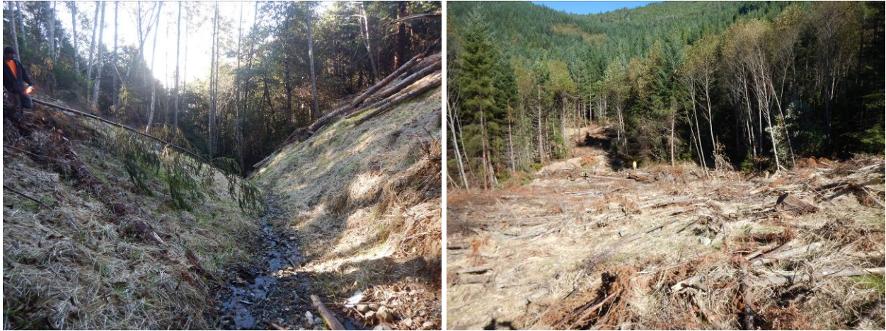
Figure 14. Photographs of YTWRD road decommissioning activities in Terwer Creek (T800 Road – Left: stream crossing removed; Right: treated road segment).
