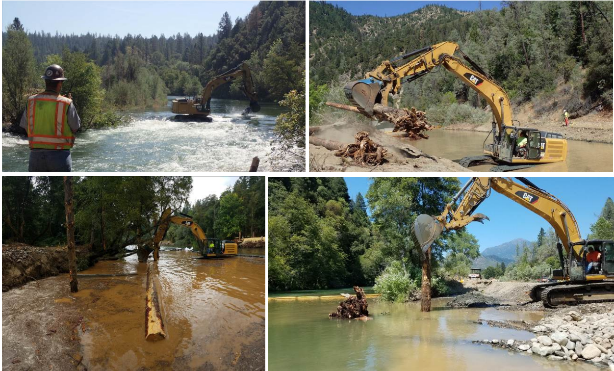
Figure 11. YTWRD crews operating heavy equipment on the Bucktail Restoration Project (Top) and on the Sheridan Deep Gulch Restoration Project (Bottom), Trinity River, California.
