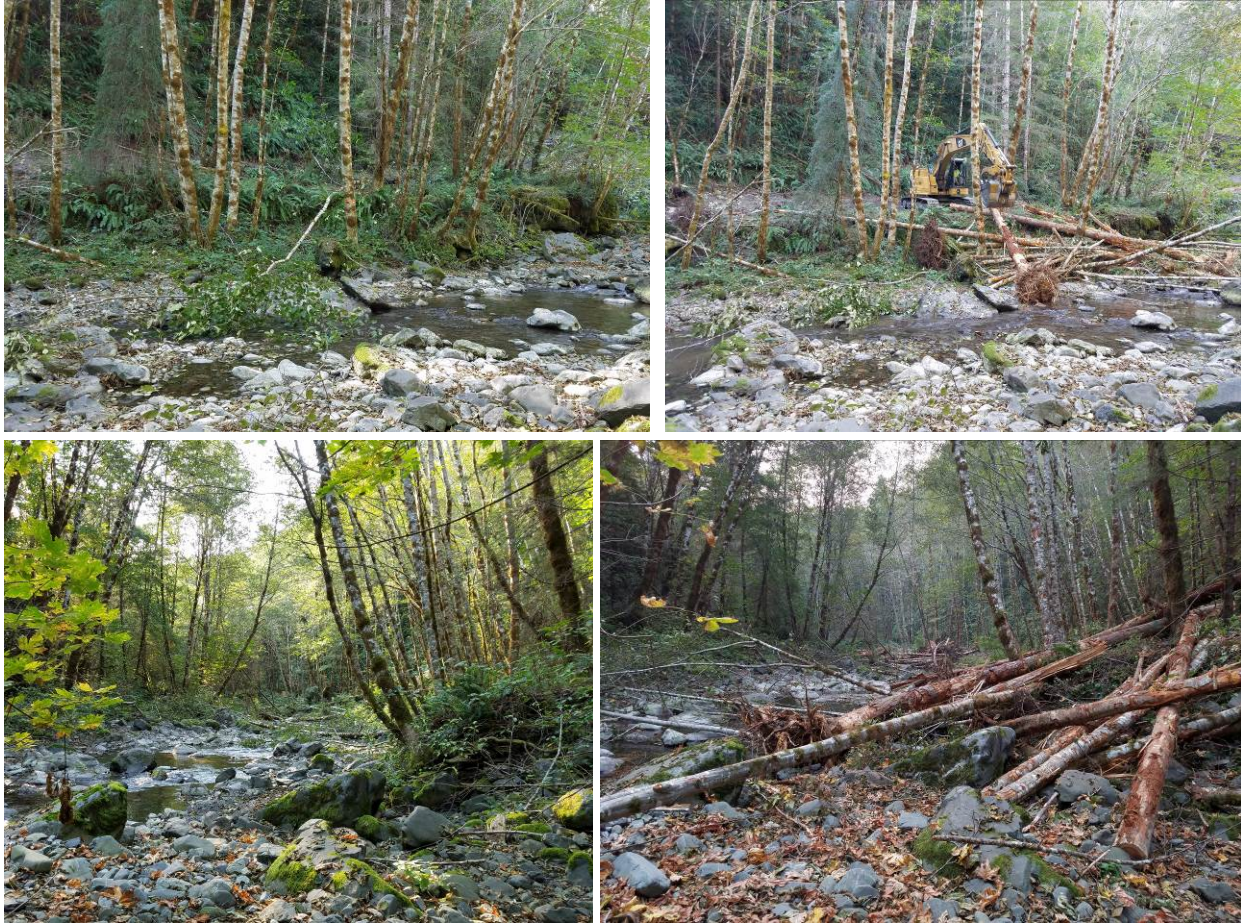
Figure 9. Photographs of wood loading in West Fork Blue Creek (Left: enhancement sites prior to wood loading; Right: the same sites during wood loading activities – 09/28/17).
