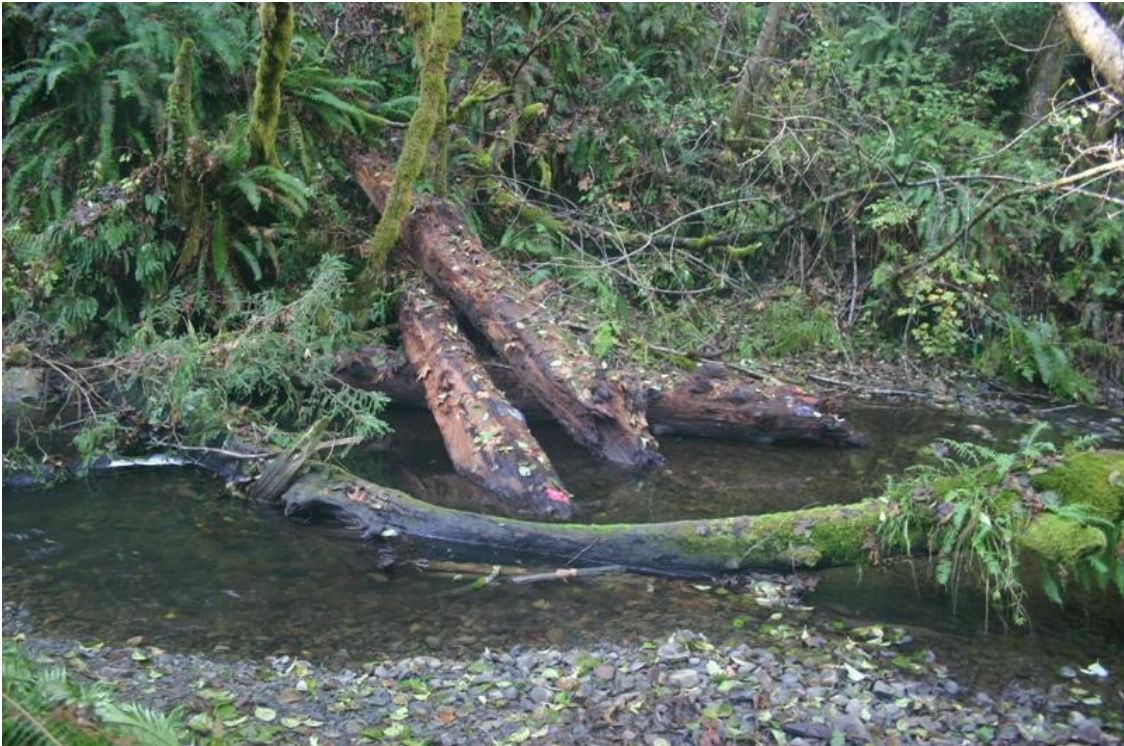
Figure 24. Shallow pool near top of project reach following installation of structure #3, Mainstem McGarvey Creek, Lower Klamath River, California, September 2008.
