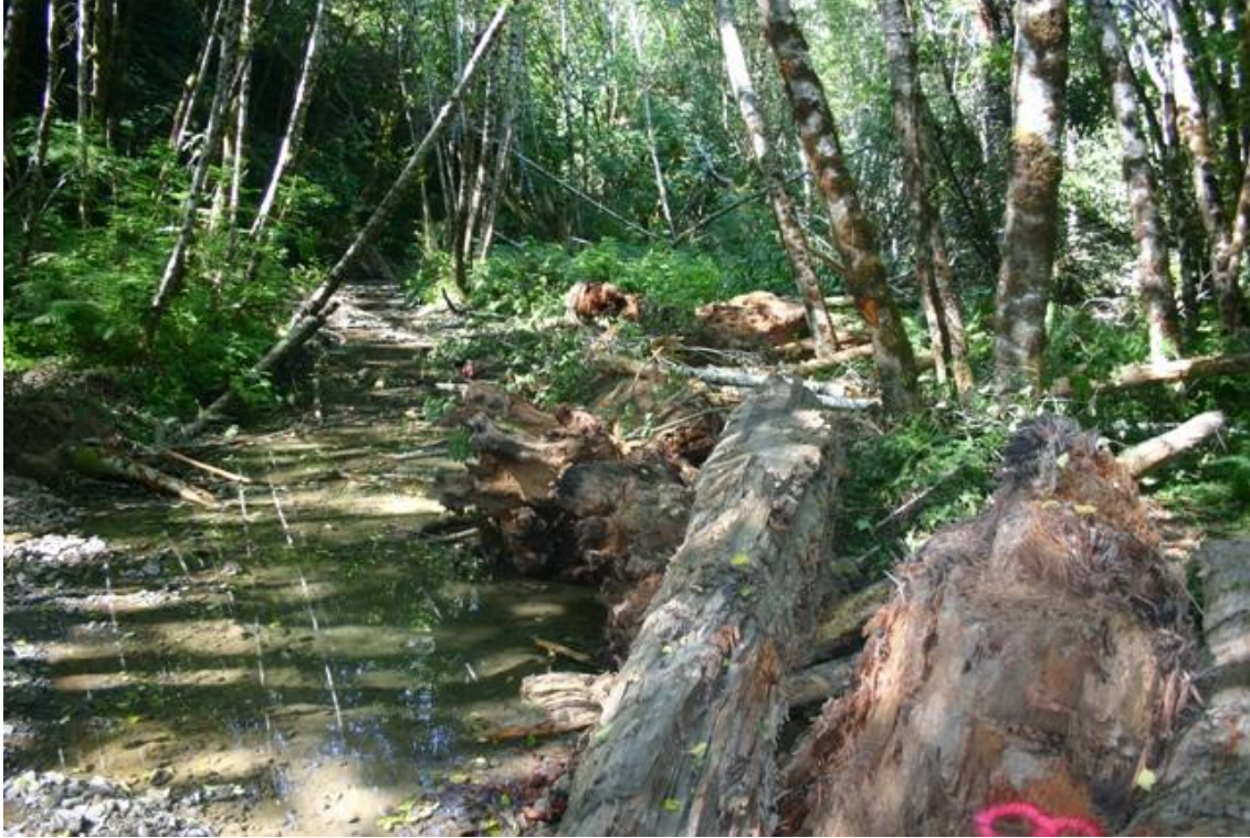
Figure 69. Step-run in middle portion of reach following installation of structures #10, Mainstem McGarvey Creek, Lower Klamath River, California, September 2008.
