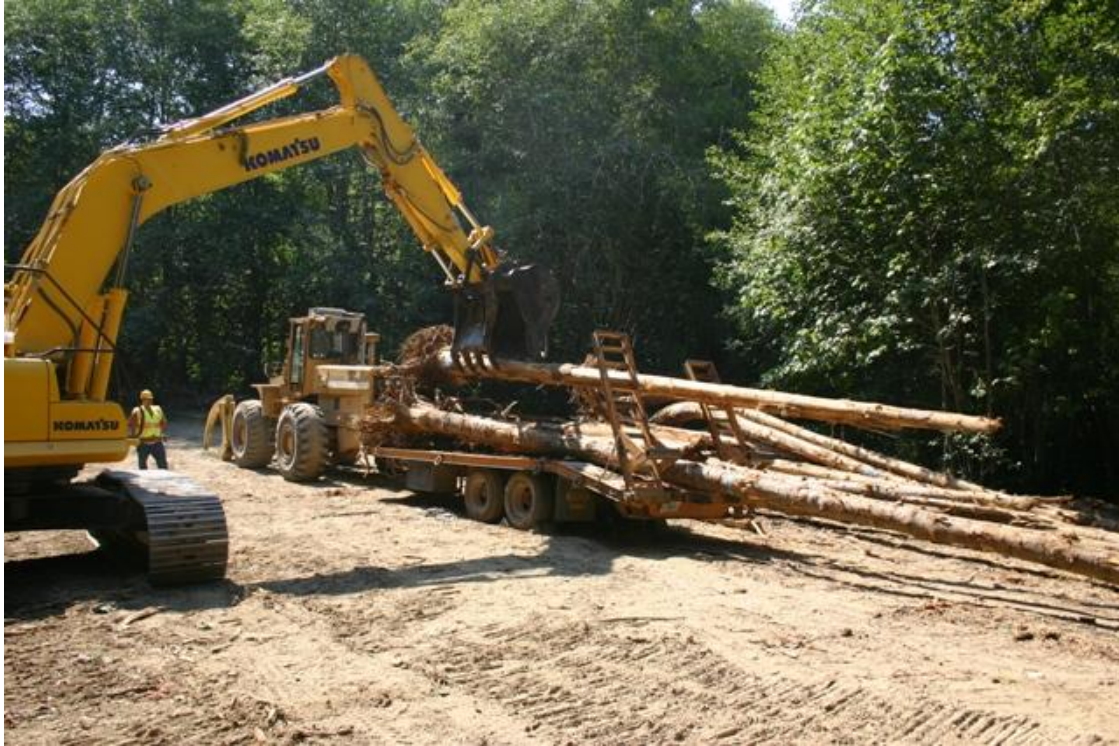
Figure 11. Salvaged LWD being loaded for transport from the stockpile area to the structure sites, McGarvey Creek, Lower Klamath River, California, 2008.
