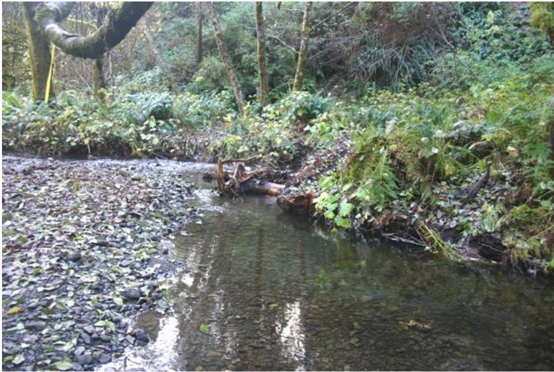
Figure 64. Backwater pool in upper portion of reach following installation of structure #7, Mainstem McGarvey Creek, Lower Klamath River, California, November 2008.
