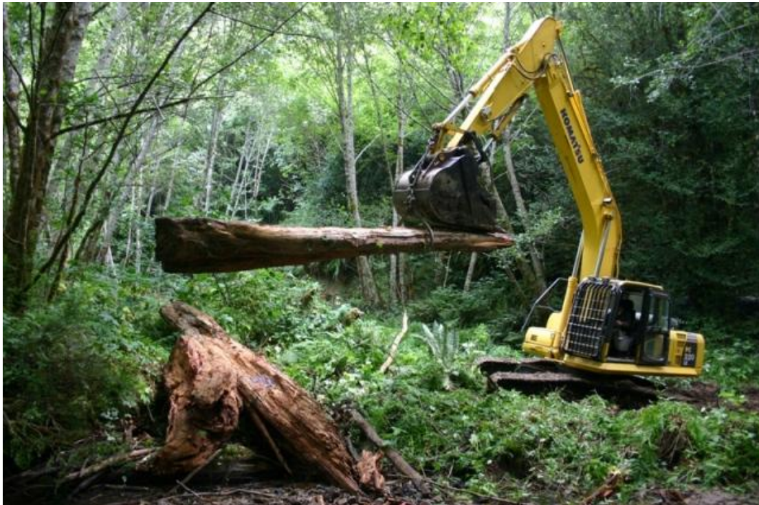
Figure 12. Excavator fitted with log grapples being used to transport LWD to structure site, McGarvey Creek, Lower Klamath River, California, 2008.
