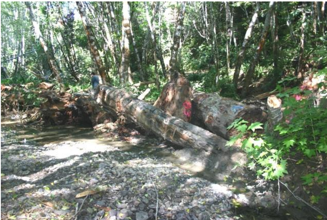
Figure 70. Step-run in middle portion of reach following installation of structures #10, Mainstem McGarvey Creek, Lower Klamath River, California, September 2008.
