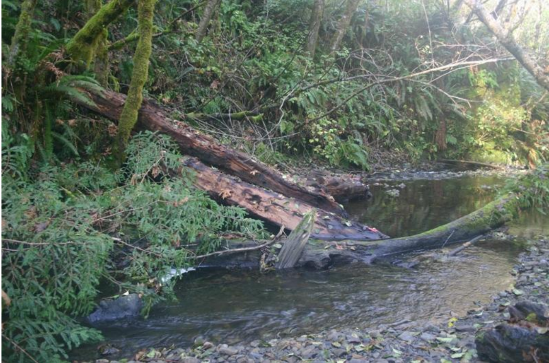
Figure 23. Shallow pool near top of project reach following installation of structure #3, Mainstem McGarvey Creek, Lower Klamath River, California, September 2008.
