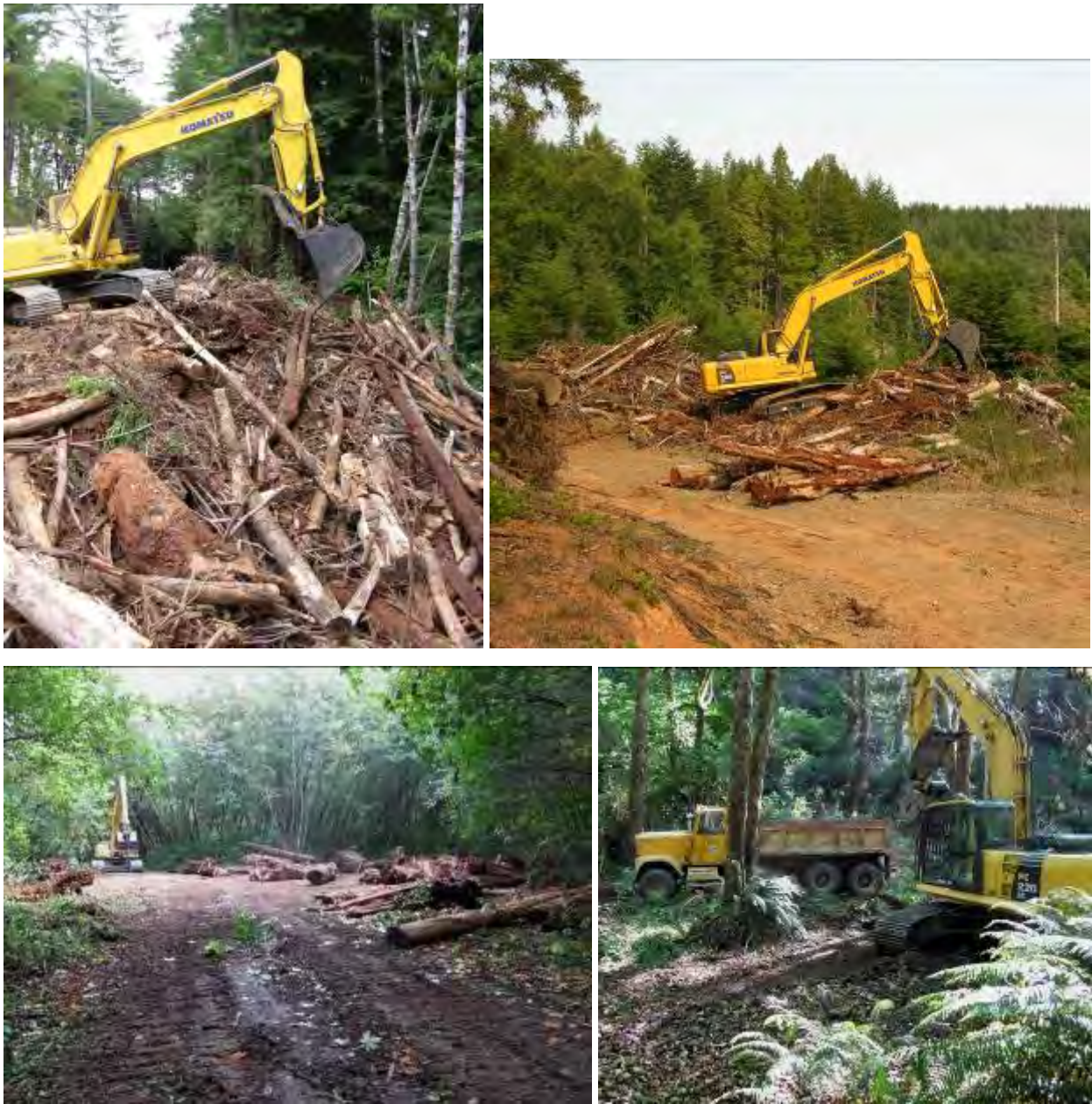
Figure 9. YTFP and Fiori GeoSciences salvaging wood from Green Diamond Resource Company lands (Top); and crews staging wood in the Waukell Creek project reach (Bottom).
