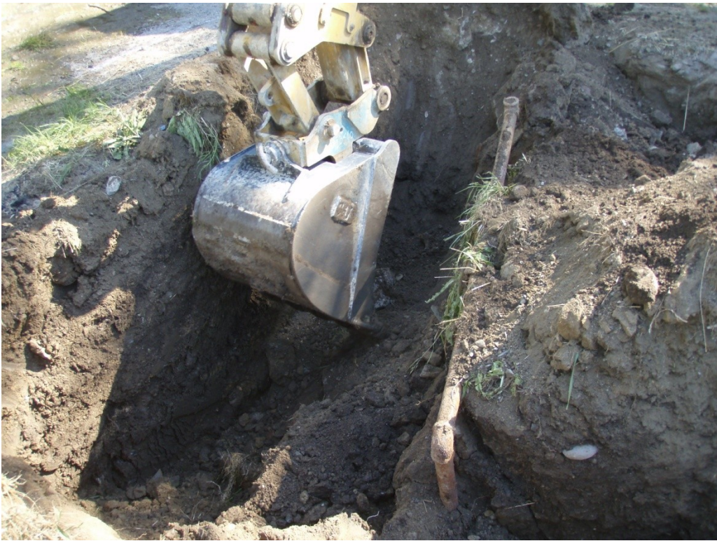
Photo 03: Removing soil from the northwest side of the UST. Note the far end of the pipe where the dispenser island was located. Direction: North
