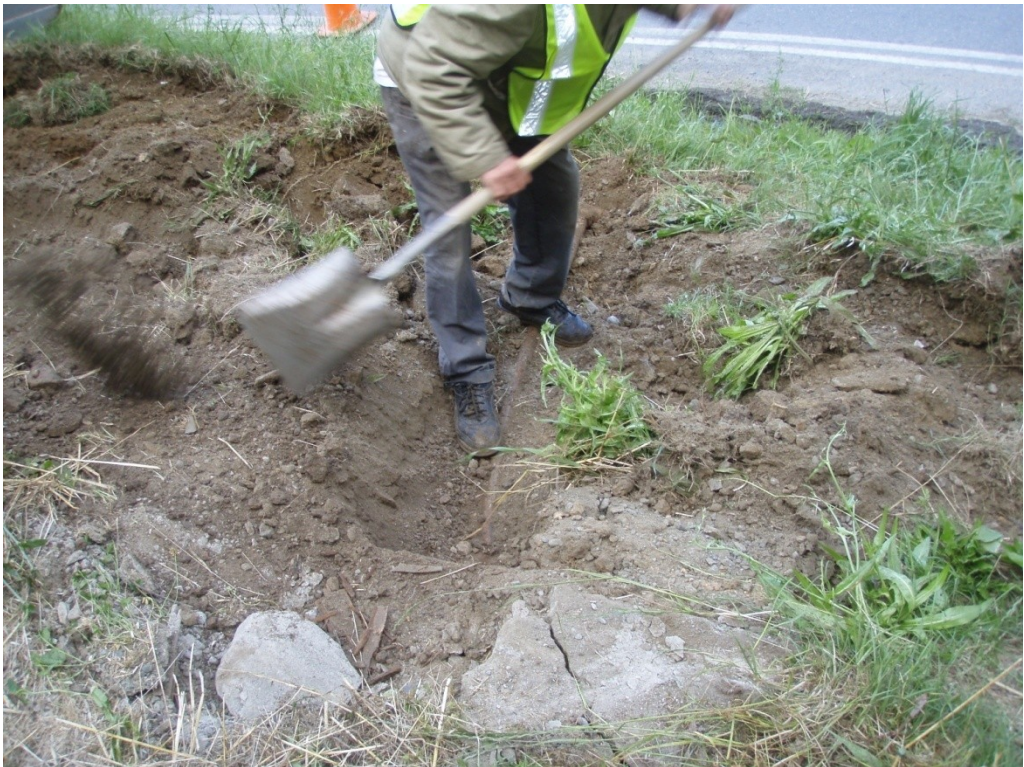
Photo 02: Uncovering the piping that connected the UST to the dispenser island (foreground).
