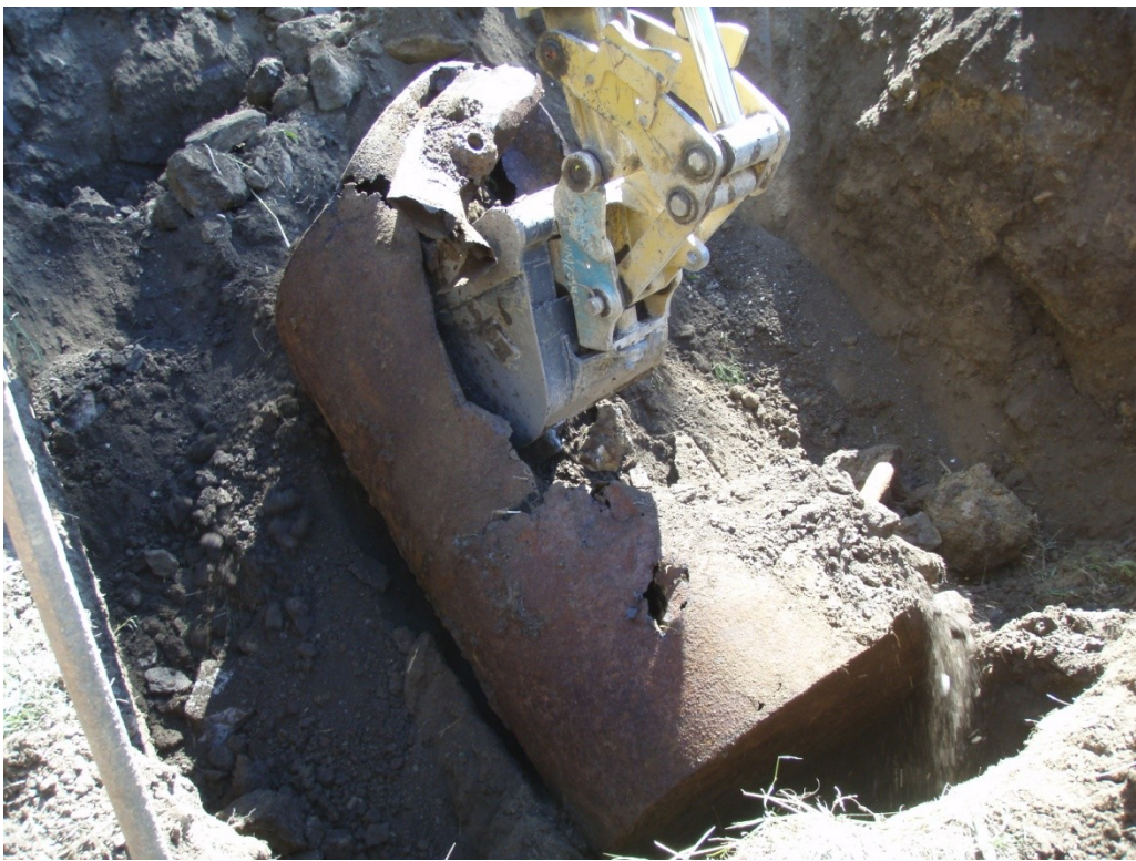
Photo 05: Removing the empty, badly deteriorated UST following removal of contents and triple rinsing. Direction: Northeast
