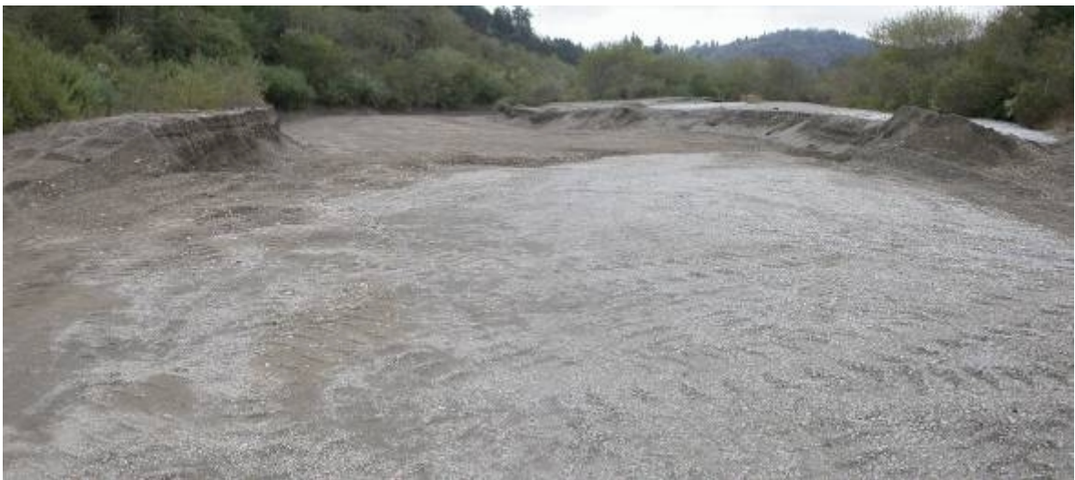
Figure 24. Photographs of the fluvial corridor of Hunter Creek during the second year of channel excavation operations, Lower Klamath River Sub-basin, California (October 2005).
