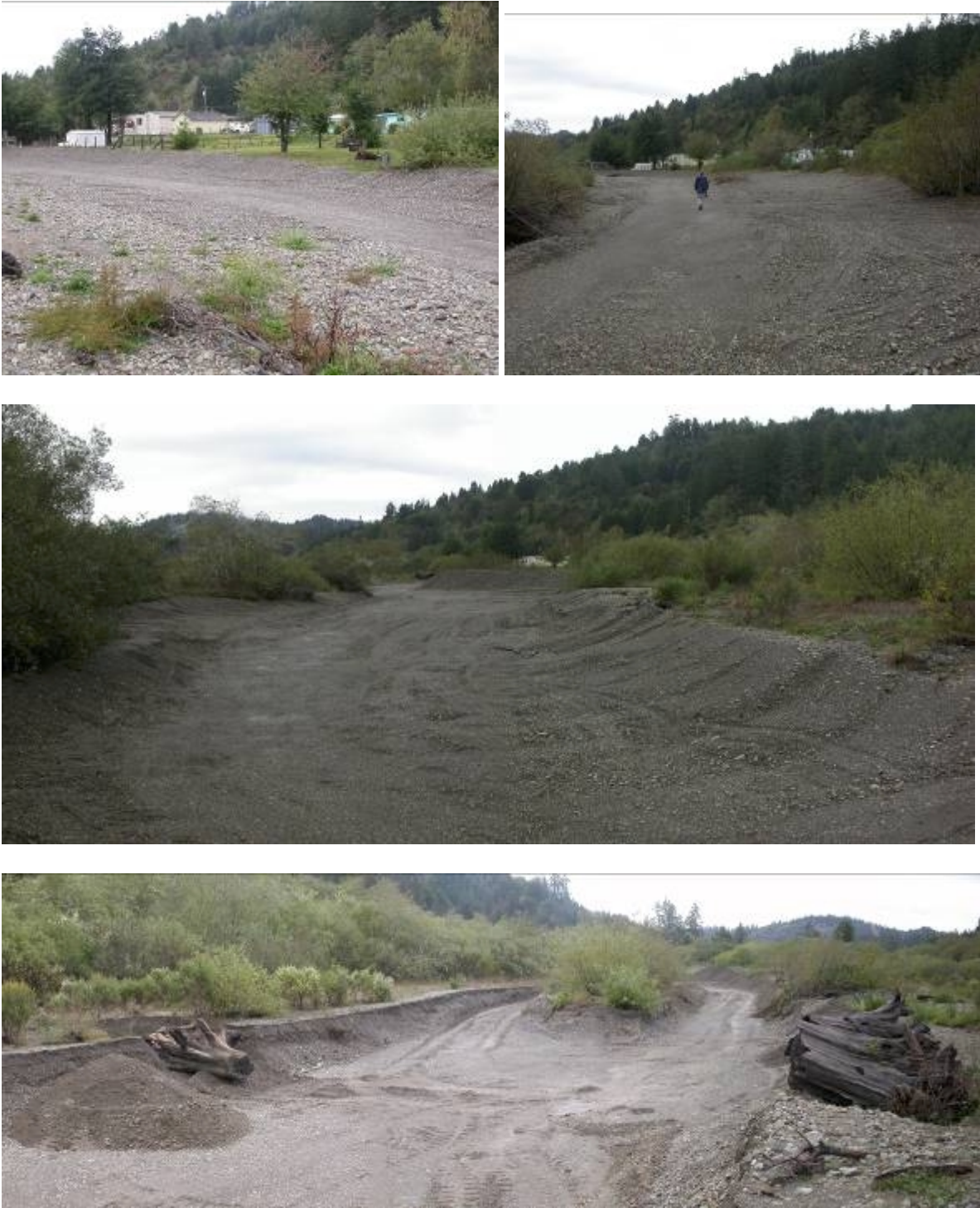
Figure 21. Photographs of the fluvial corridor of Hunter Creek during channel excavation operations, Lower Klamath River Sub-basin, California (Late October 2004) (Note the white house located in the top three photographs).
